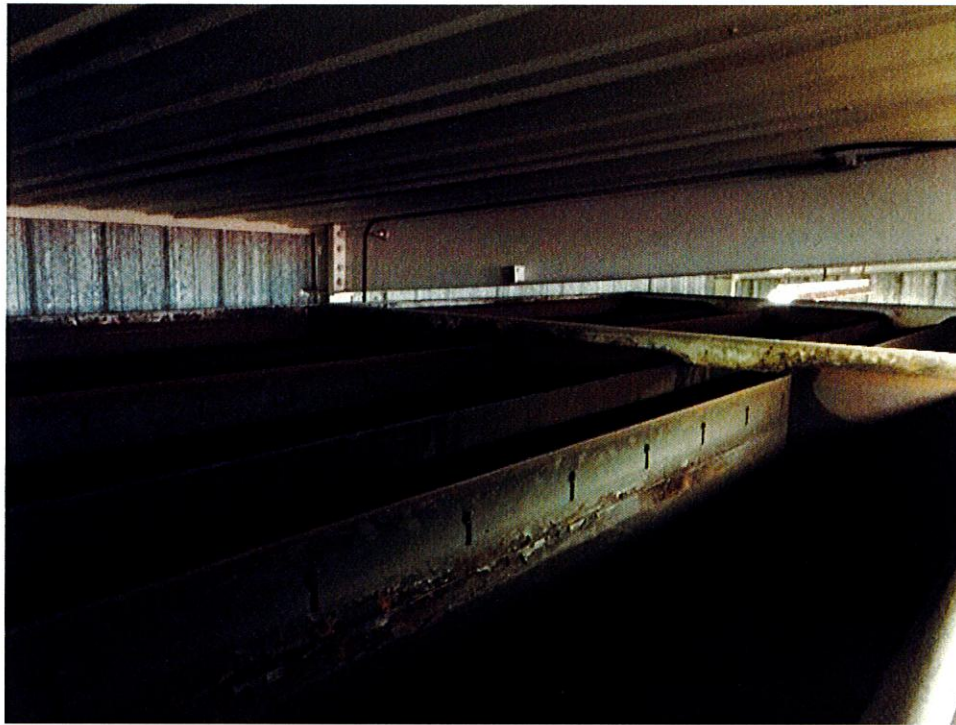
Manganese Greensand Gravity Filter Unit
