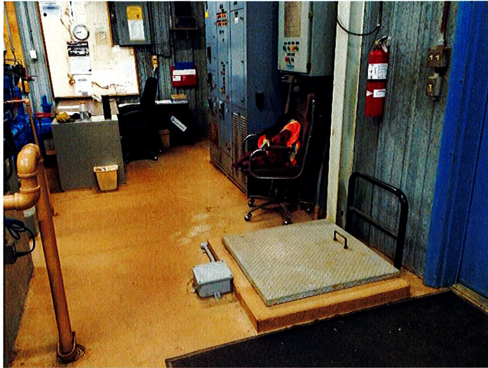
Reservoir Access Hatch
