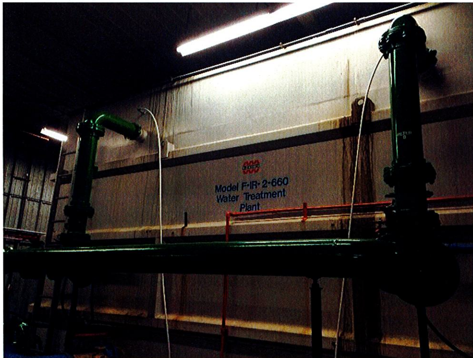
Manganese Greensand Gravity Filter Unit
