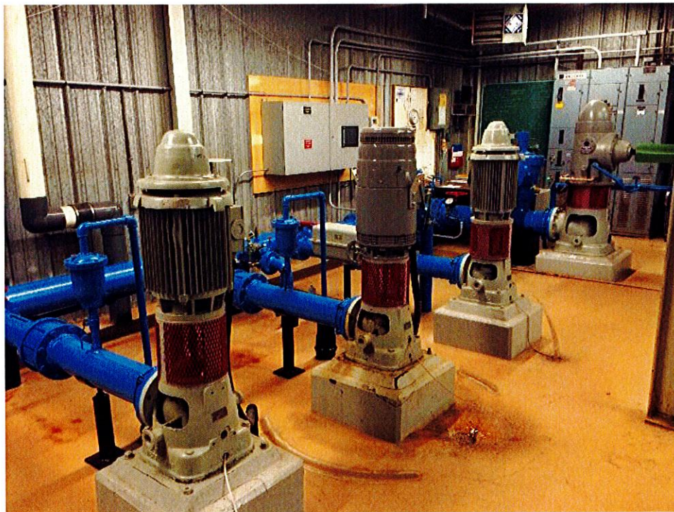
Distribution Pumps and Header
