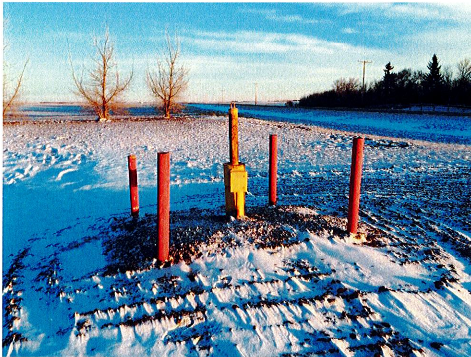
Well #3 Well Head
