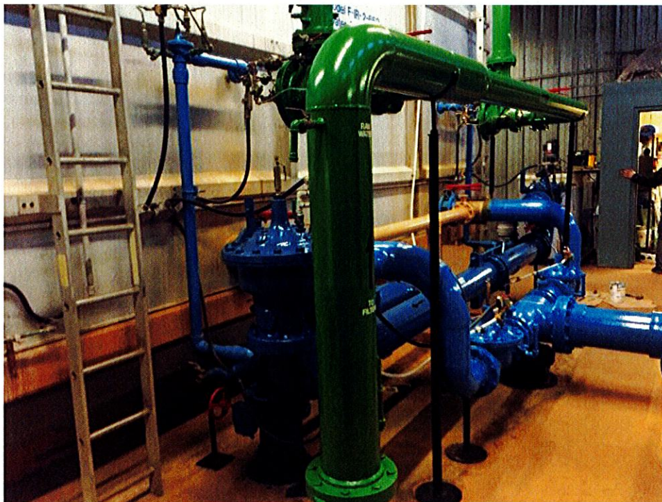
Filter Process Piping
