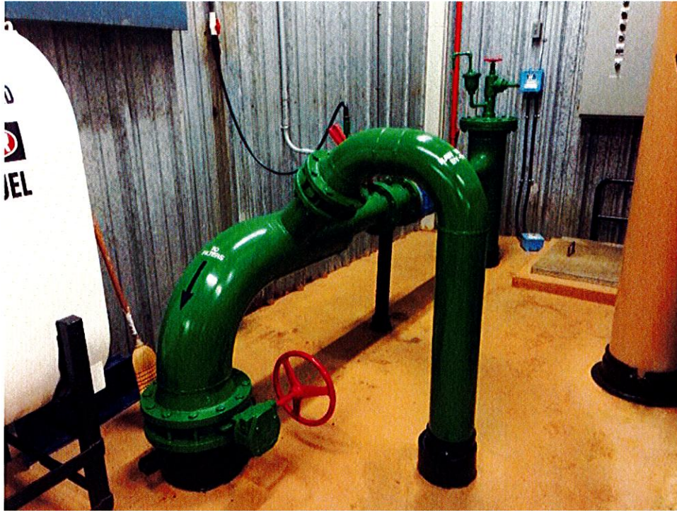
Raw Water Influent Piping
