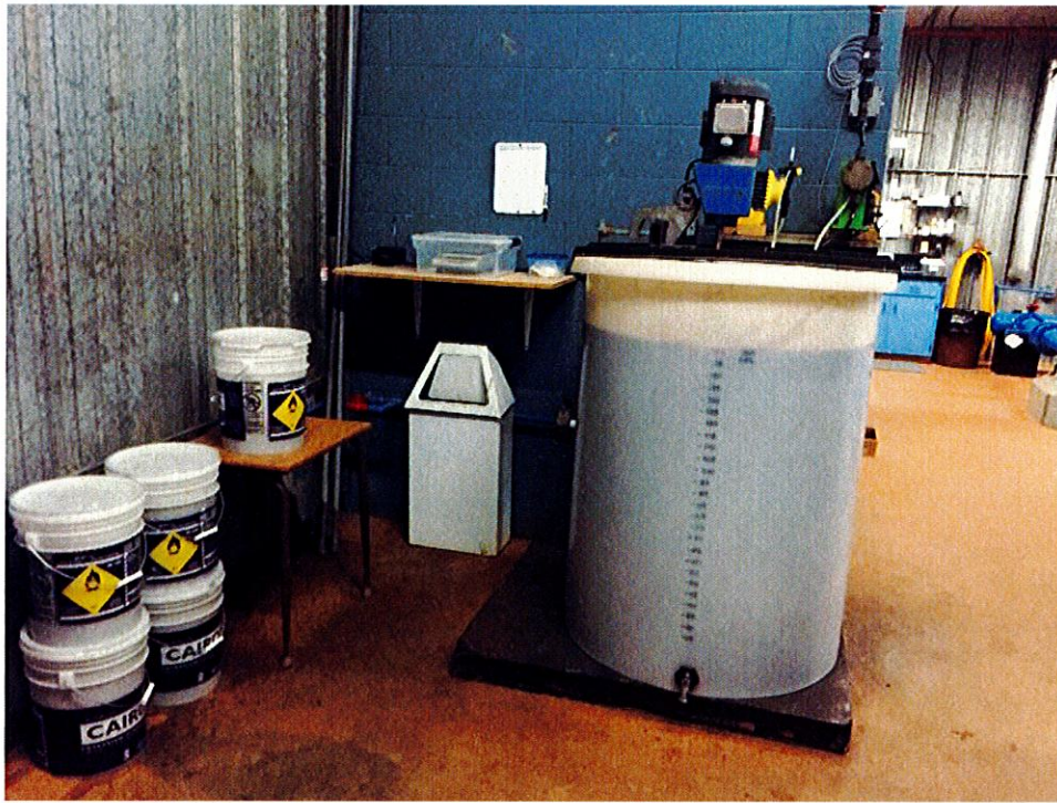
KMnO 4 Feed Station
